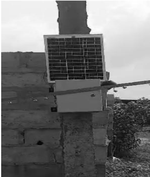
Figure 8: Field deployment of the solar-powered bird repeller system mounted directly onto an active overhead distribution pole corridor
